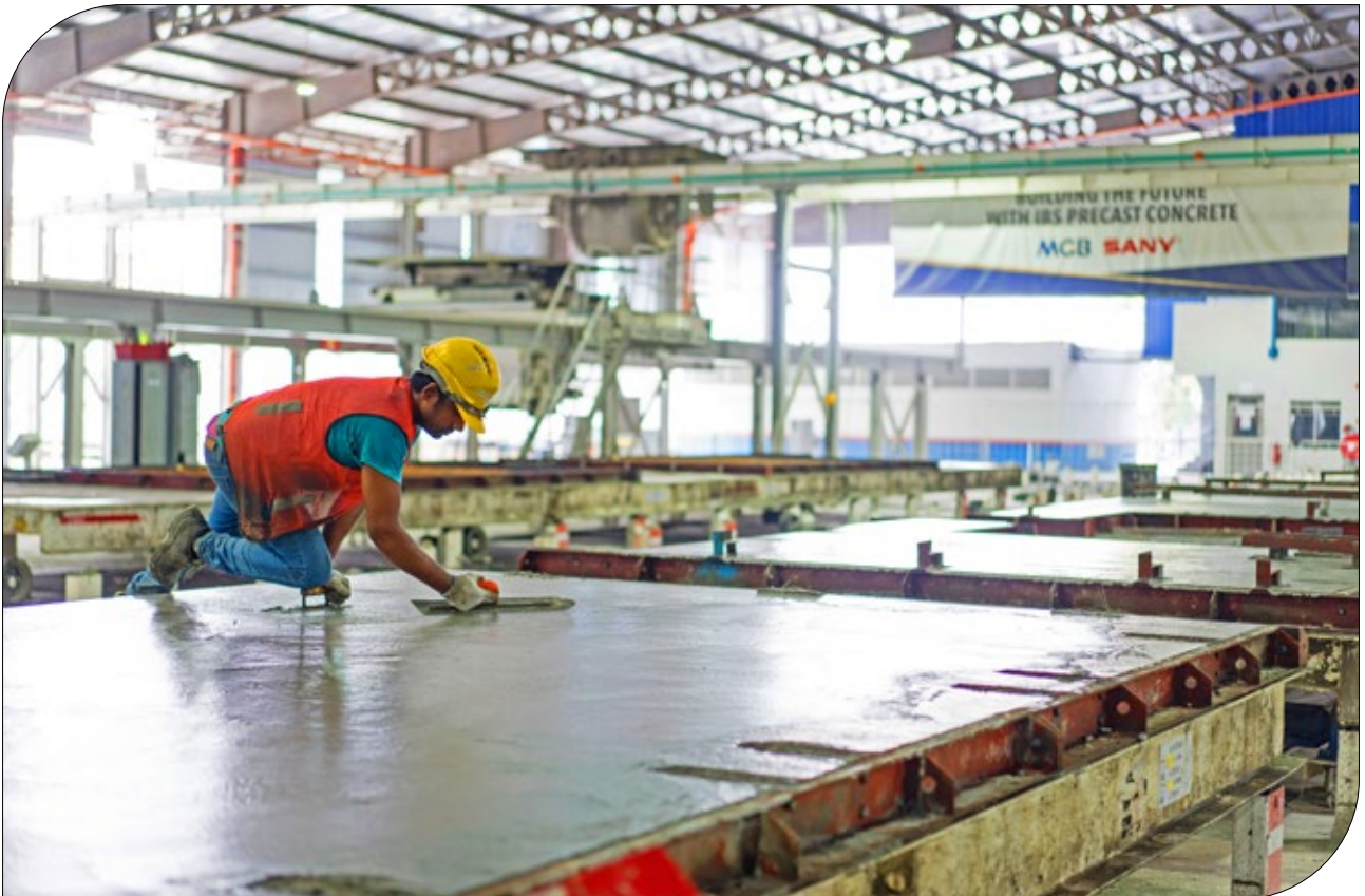
Industrialised Building System ("IBS") Precast Plant at Nilai
